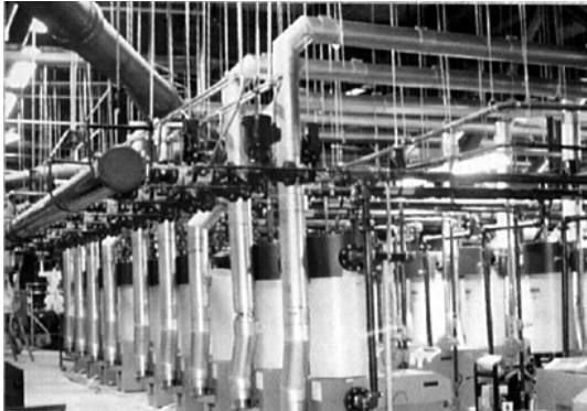
A wide range of materials for inner liners and outer shells are available with Schebler chimneys. In this application, special high-corrosion-resistant stainless steel was used to vent 38 high-efficiency boilers in a large sports complex.
